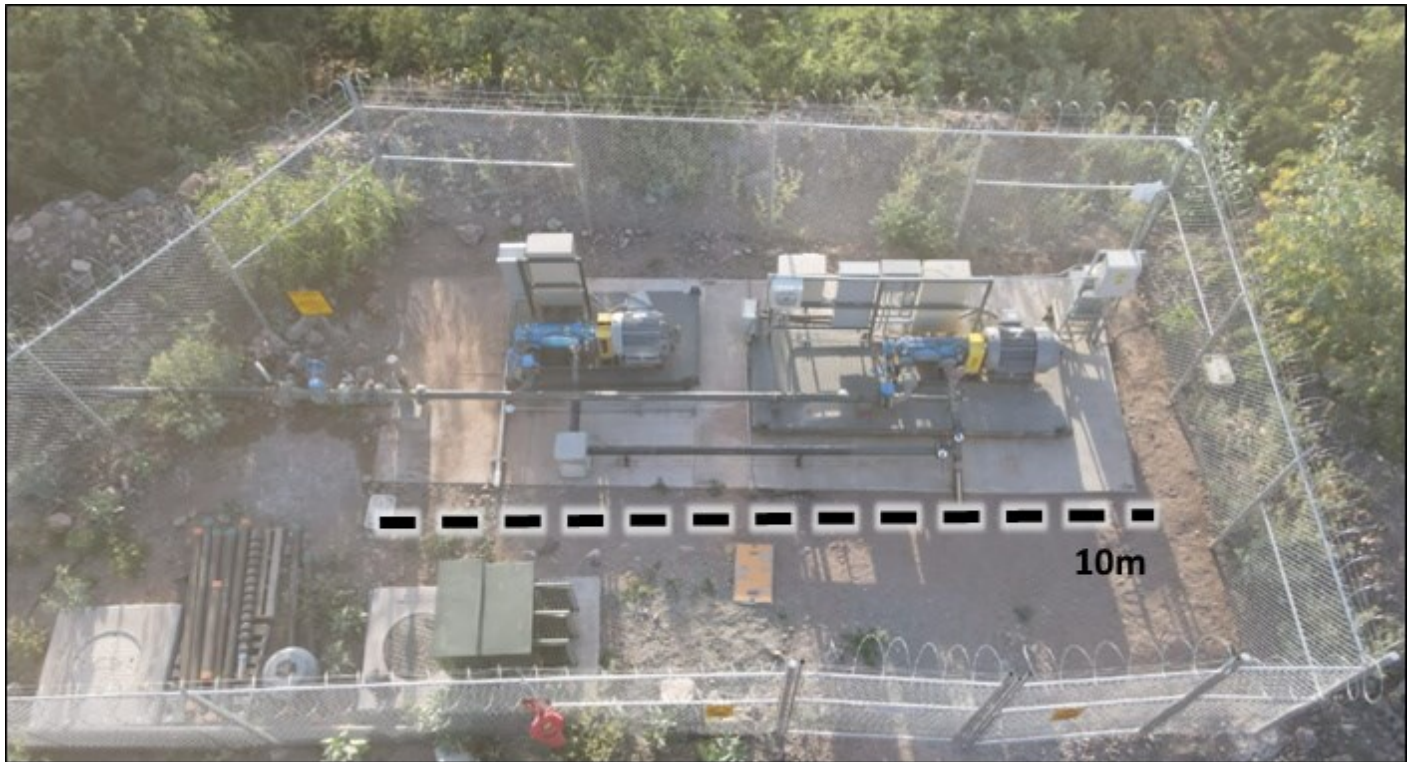
Figure 4-3: Sonora River Pumping Station
