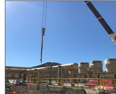
Merrill-Crowe Solution Pumps
