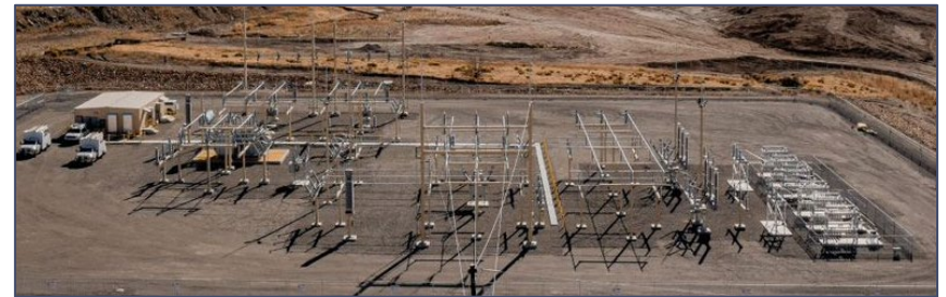
Completed NVE Substation
