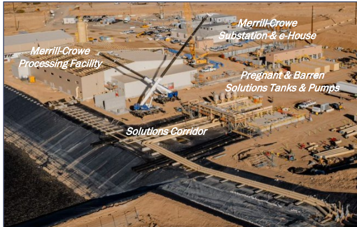
Merrill-Crowe Plant, Solutions Corridor, Substation
