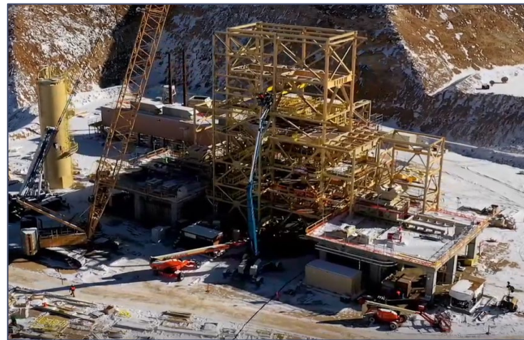
Tertiary Crusher Area
