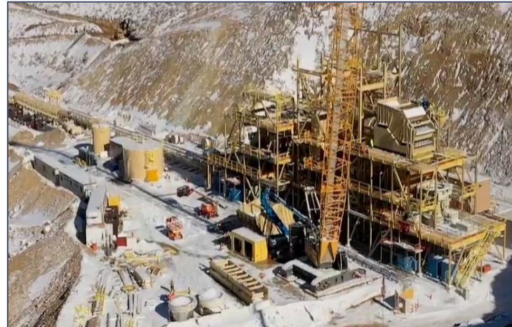
Secondary Crusher Area
