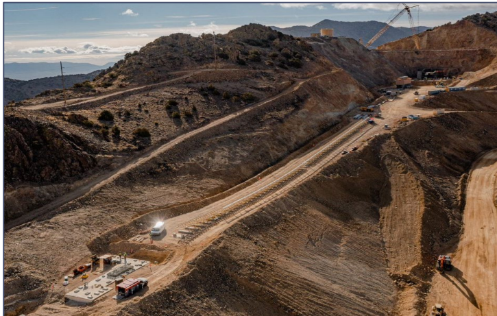
Primary Crushed Ore Conveyor
