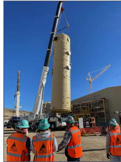
Merrill-Crowe De-aeration Tower
