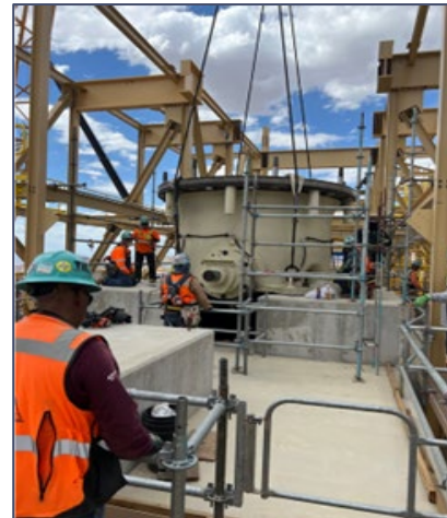
Secondary Crusher Rough Set
