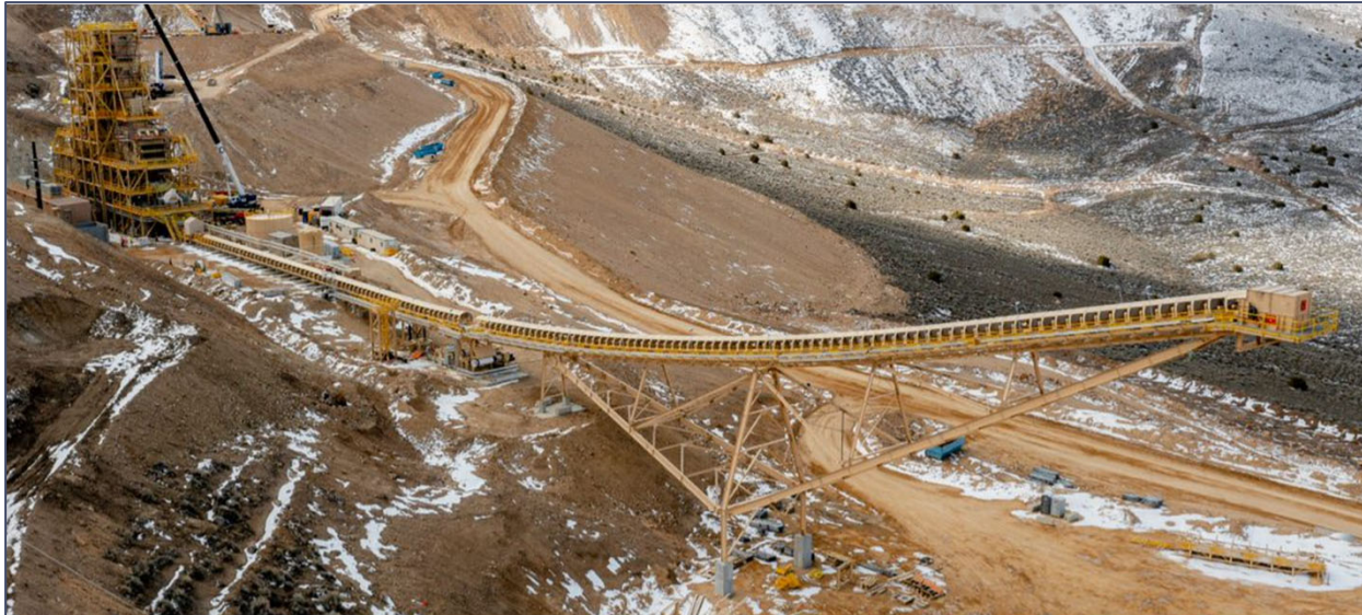
Secondary Crusher & Primary Stacker Conveyor
