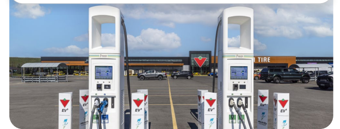
Electric vehicle charging stations at a Canadian Tire Store – Welland, Ontario
