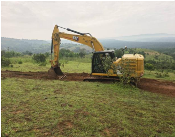
Access road preparation to test pit 05 at the north box cut waste rock dump
