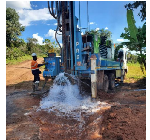
Production water borehole drilling at Kabanga Site, 132m deep, providing a yield of 28,000 L/H
