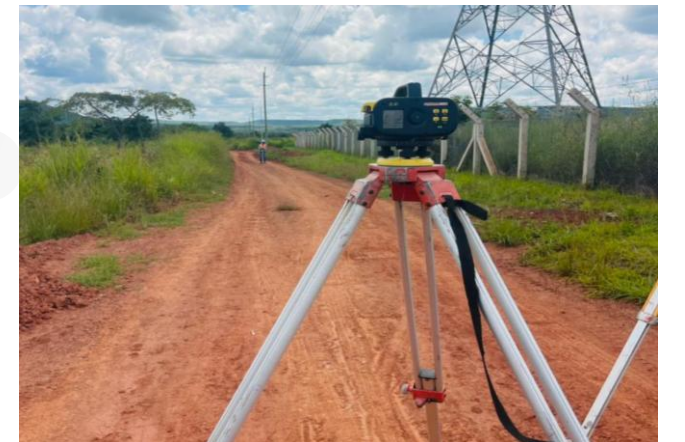
AGS leveling task through the 220Kv transmission line to determine the ground profile for angle point No.29 at Nyakanazi substation
