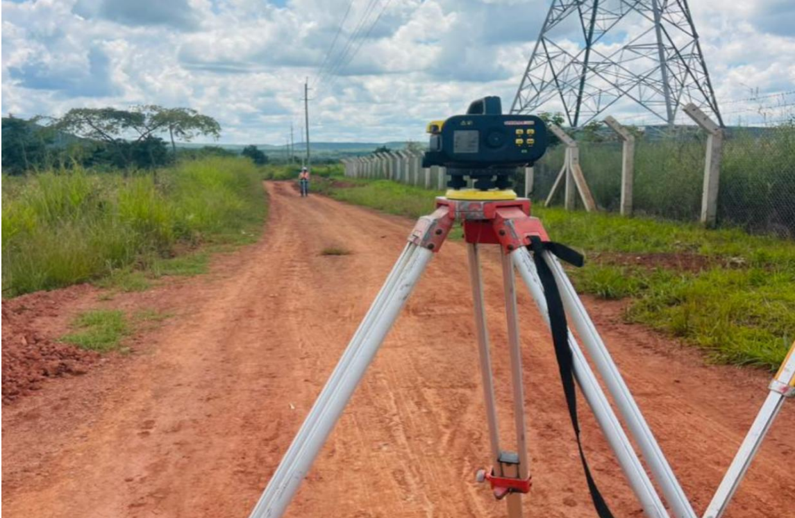
Figure 5: AGS leveling task through the 220Kv transmission line to determine the ground profile for angle point No.29 at Nyakanazi substation
