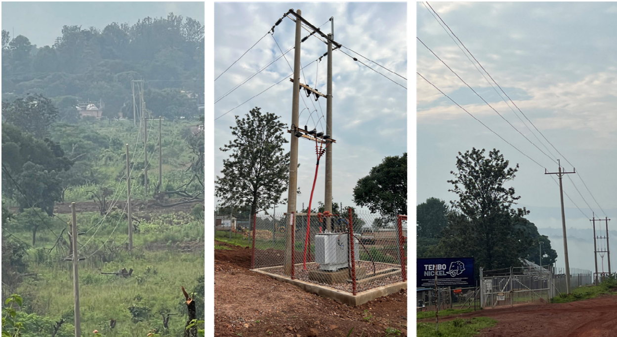
Figure 2: Images of the 33-kilovolt power line connecting the Kabanga Nickel Project operations camp, located on the Special Mining Licence, to the regional power grid.
