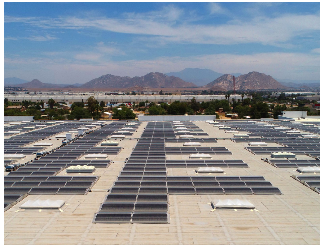
Perris, California, Distribution Center
