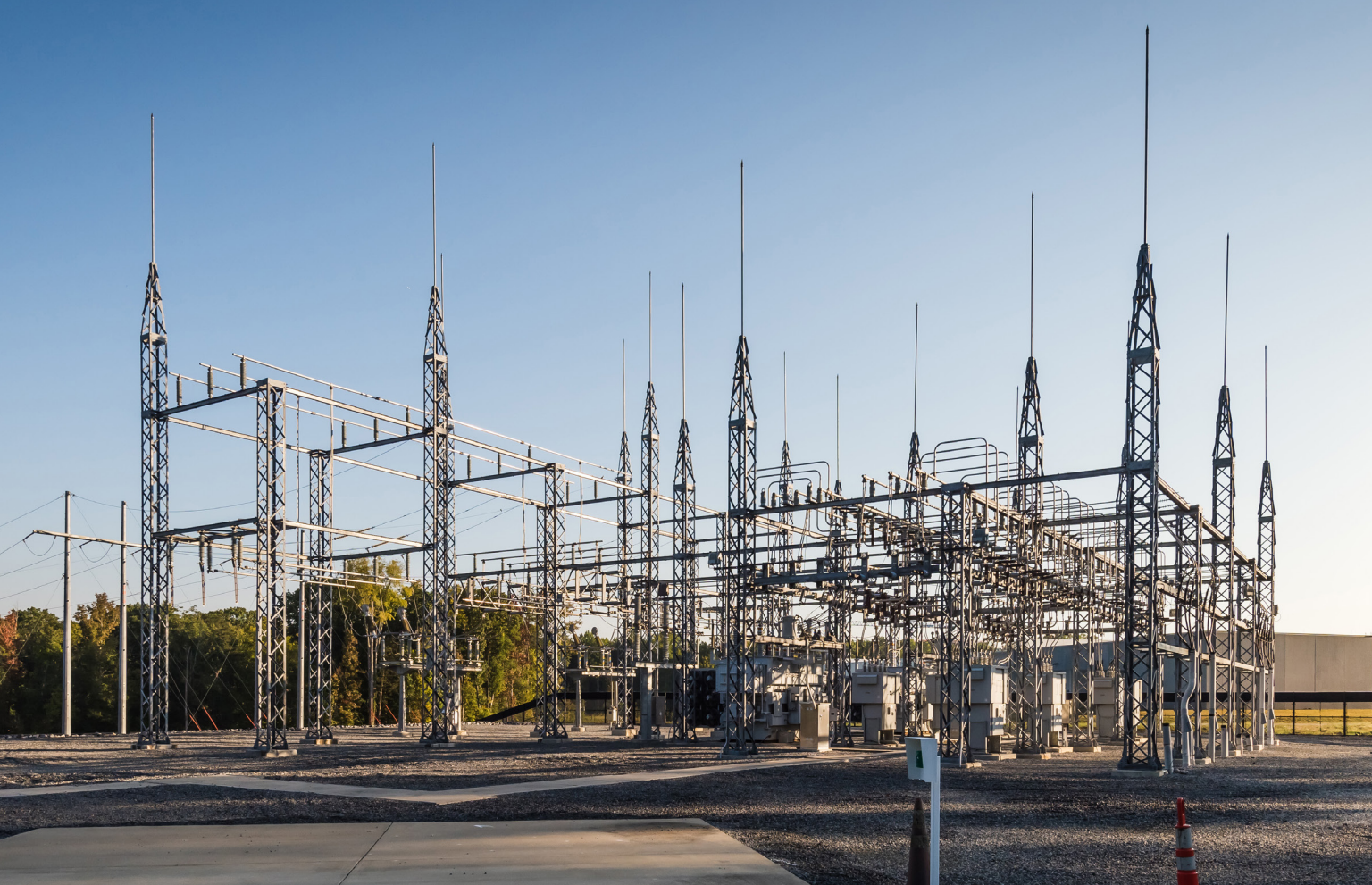
Self Healing Grid Substation
