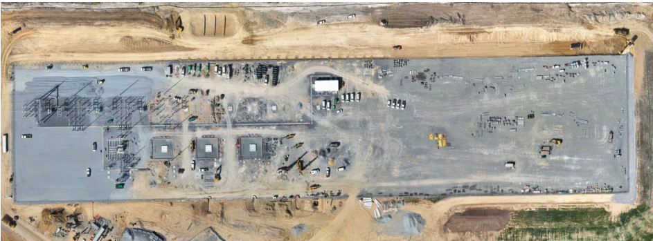
Substation to support $5 billion Wolfspeed semiconductor manufacturing facility in North Carolina
