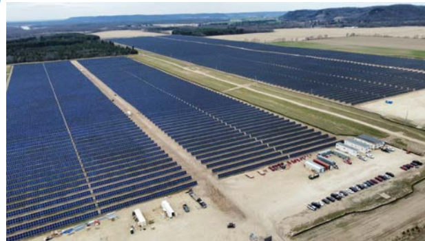
Bear Creek – 50 MW project
