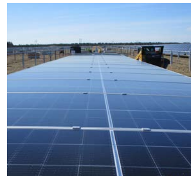
Wood County – 150 MW project
